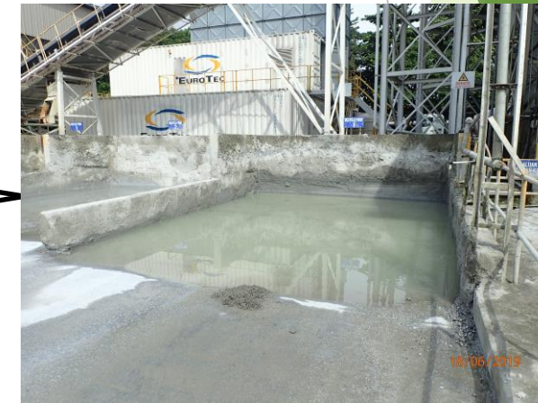
The reception ponds are where the trucks wash their bowls out and discharge the water and waste into these wedge pits. The front end loader operator frequently cleans these pits and dumps the material into the Material Drying Pits.
