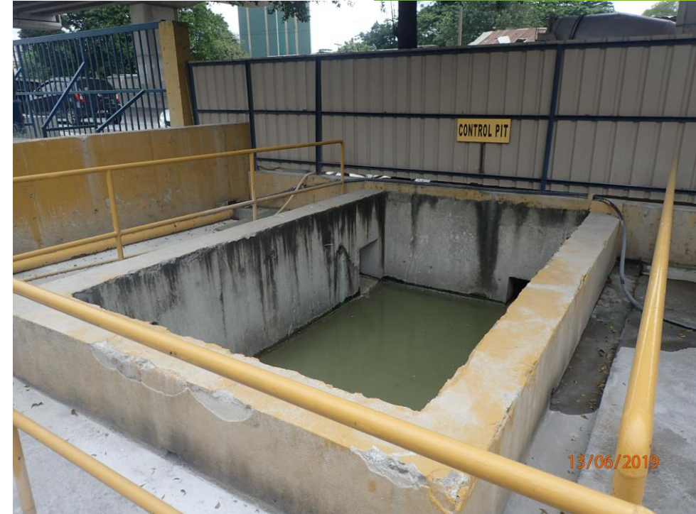
Control Pit designed to capture the water and settle out the suspended solids from Clean area pavements
