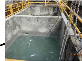
R1 & R2 are the recycled water pits where the water is stored before being pumped and recycled to be used as batch water in the concrete.
