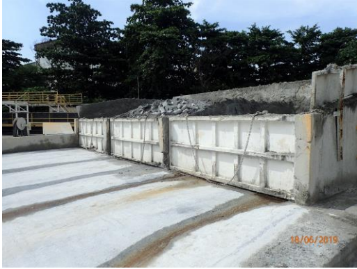
Material Drying pits where the sludge from the reception ponds, sediment ponds and S1 & S2 are removed by the front end loader and placed to dry out before being transported away by truck.
